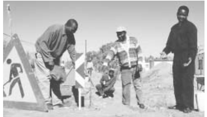
Asakheni Construction, emerging contractors in Mpumalanga, install a stormwater drainage system. With the help of a guarantee of R96,491 ($12,061) from MEEC, the contractors obtained a bridge loan to initiate a R964,912 ($120,614) government project. ("Asakheni" means "let us build" in the Ndebele language.)
